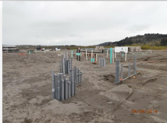
Electrical Conduits to main electrical room
